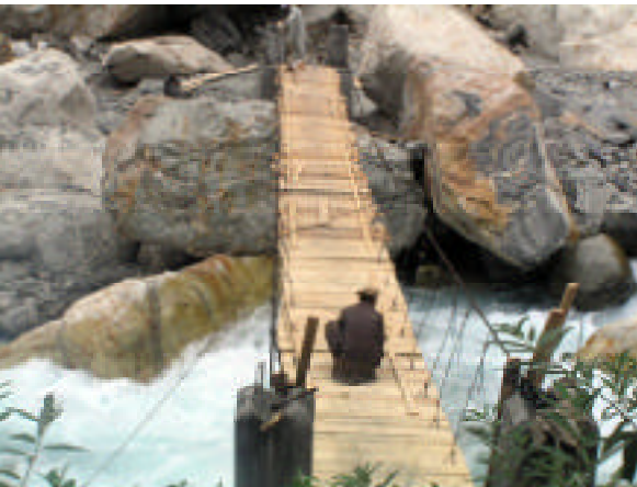
Dubair Bela bridge for pedestrians, under construction, below - completed by OAKDF early October
